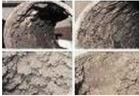
Fig.5.4: Scales Formed Due to Corrosion
